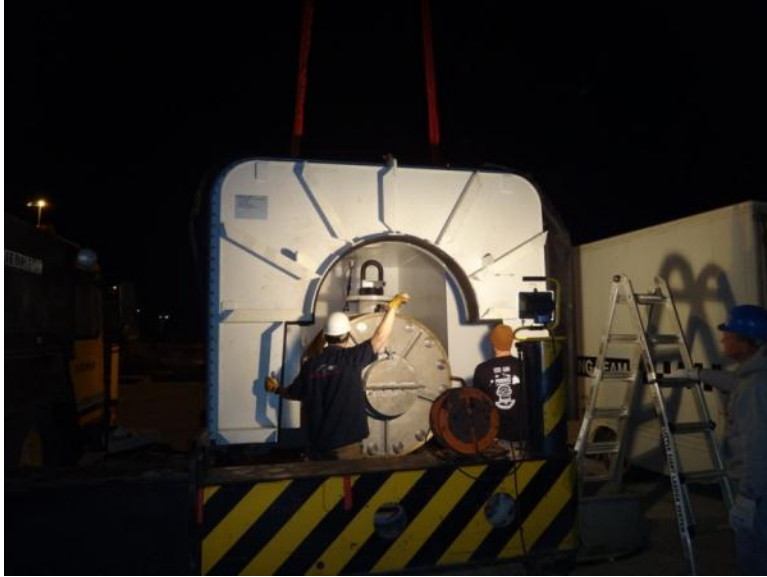
The cofferdam being lowered onto the ready-for-issue hub in preparation for reinstalling hub on the shaft.
