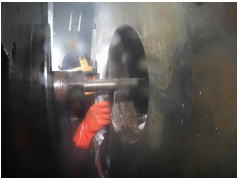
Underwater Repair Specialist completing the removal of the hub (on left) from the shaft.
