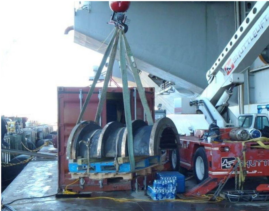
A portable crane is used to move bottom bearing shell from the dive and rigging barge to the pier.
