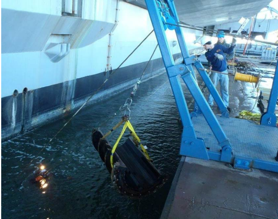
With a Phoenix diver watching from the water, the repair crew pulls one-half of the stern tube bearing clear from the water at the starboard side of the USS GEORGE H. W. BUSH using A-Frames (blue structure) and hydraulic tuggers (not visible).
