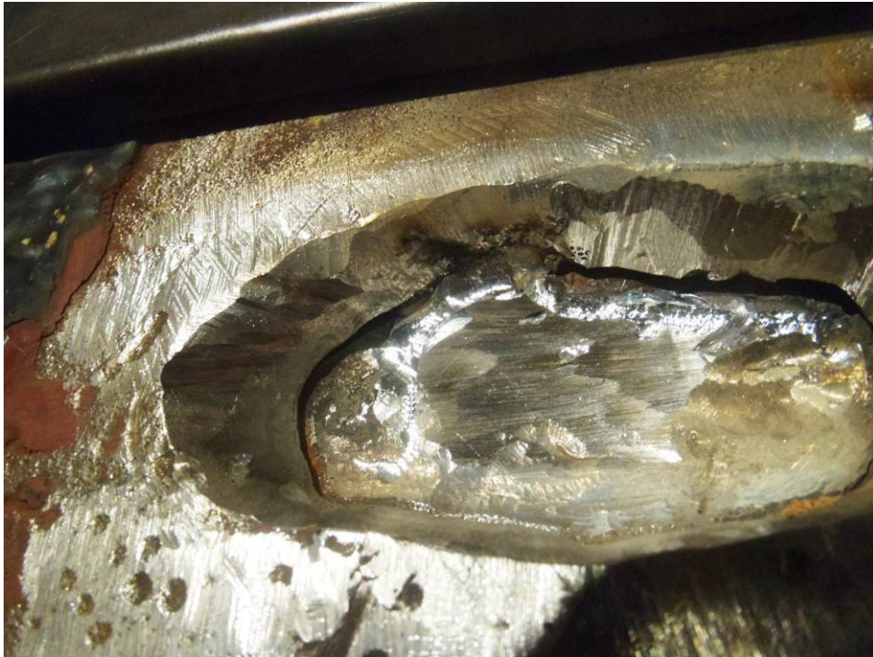
An example of a crack that has been ground out and the backing plate before welding commences.
