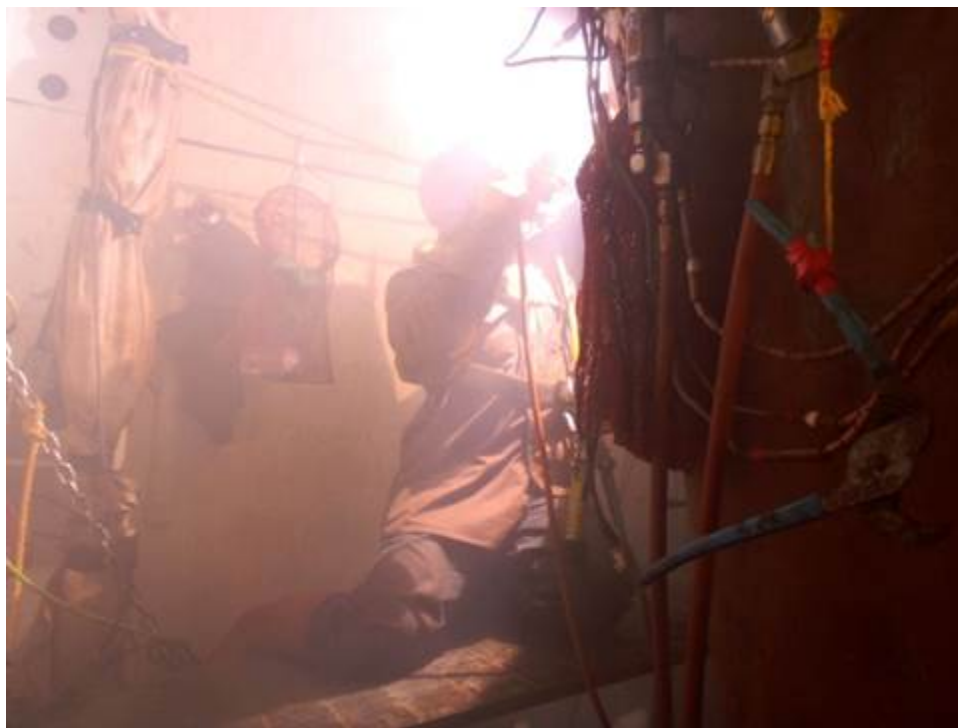
A Phoenix diver inside a hyperbaric dry chamber – habitat - performing a weld on a Navy ship. The procedure for aluminum hulled ships involves using a Gas Metal Arc Welding (GMAW) process.
