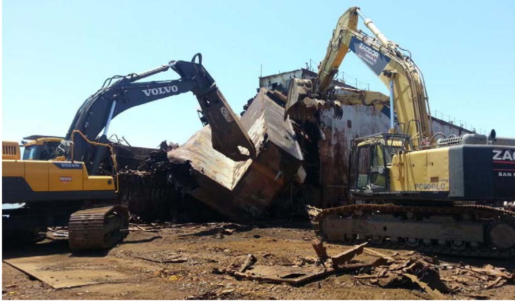
Titan's excavators equipped with metal shears and gripping claws tear into a mid-body overhang on one end of the dry dock. Removed material is sorted and loaded on trucks for scrapping.
