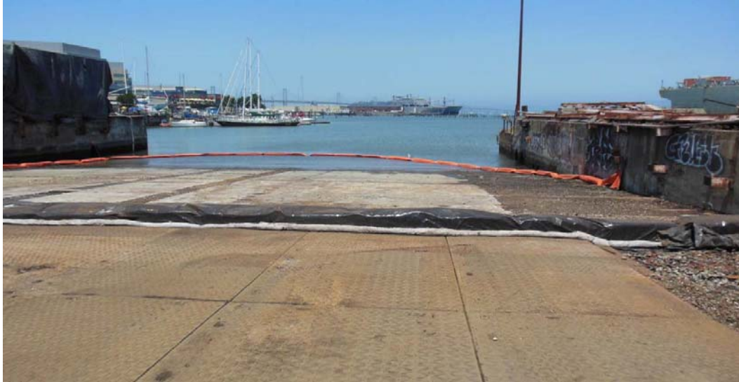
Crane Cove dismantling site. Preparations here included sweeping the site clean, a complete covering with a geo-tech barrier and placing dura-base mats on top to protect the barrier. Note the floating boom in the background to contain any possible runoff.
