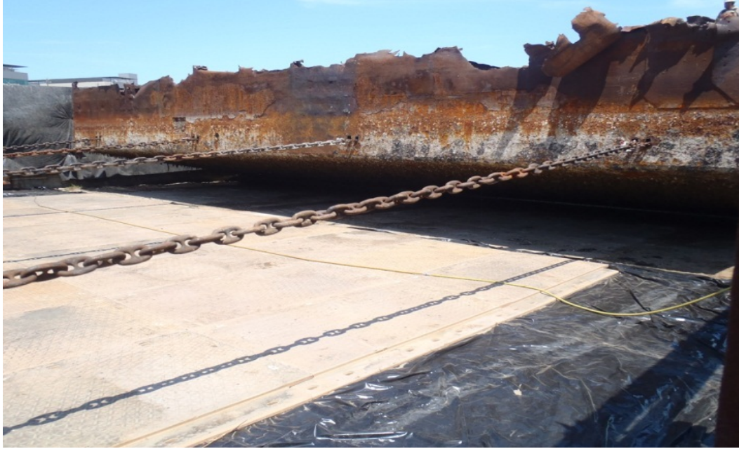
Dry dock end section, approximately 98 x 120 feet being pulled onto the Crane Cove dismantling pad. 1.5 meter diameter air bags were placed ahead of the hull to reduce friction while moving it up slope.
