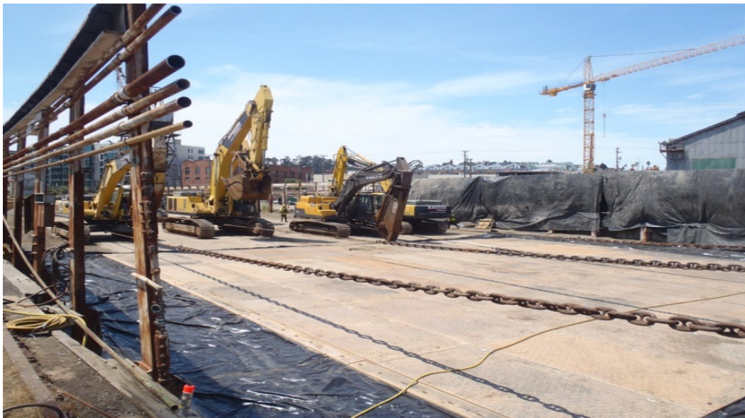
Excavators lined up at the Crane Cove dismantling site. Six of these tracked machines were used to pull the dry dock end sections onto the dura-base mat for dismantling.
