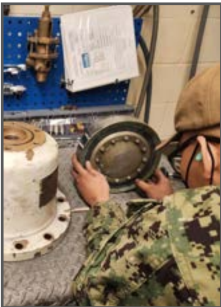
MM3 John Rabanes is inspecting the gasket of the relief valve seat. (Photo by Kirk Jeppson.)
