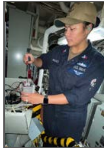
EM1(SW/AW) Jennylyn Armanza, a NAMTS Outside Electrical NEC holder, is changing out a power supply for the ship's vent fog precipitator in preparation for USS Boxer's upcoming Light Off Assessment. (Photo by Rizalito Antonio.)
