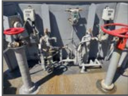
Even though the anchor windlass controls are relatively protected, they still see a significant amount of corrosion. The lines, piping and stanchions were wrapped with Mil-Spec corrosion inhibiting material then received a coating of polysiloxane paint.
