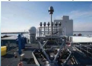
Satellite Communications Deck
