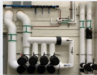
Water & dry air services
