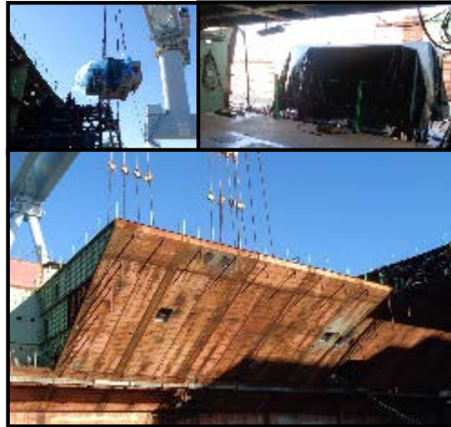
EMALS Motor Generator being loaded into Super-lift
