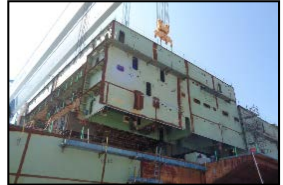
“Mega-lift” Unit 5616 – Example of build strategy improvements in action. This single CVN 79 Mega-lift required 19 separate lifts on CVN 78, greatly improving CVN 79 construction efficiency.
