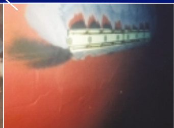
Typical anode. The flaming pattern above the anode is a normal bleaching on hull coating systems.
